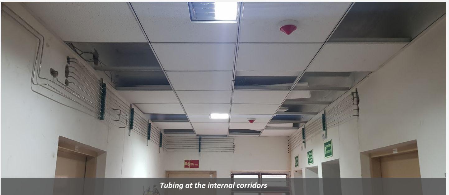
Tubing outside the lab complex
