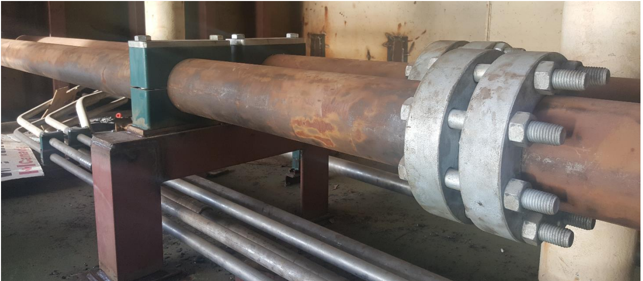
View of the 5" Sch160 pipe for the main pump lines
