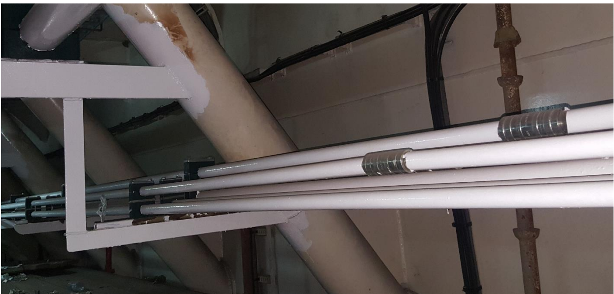
View of the small bore lines connected by Pyplok® and supported
