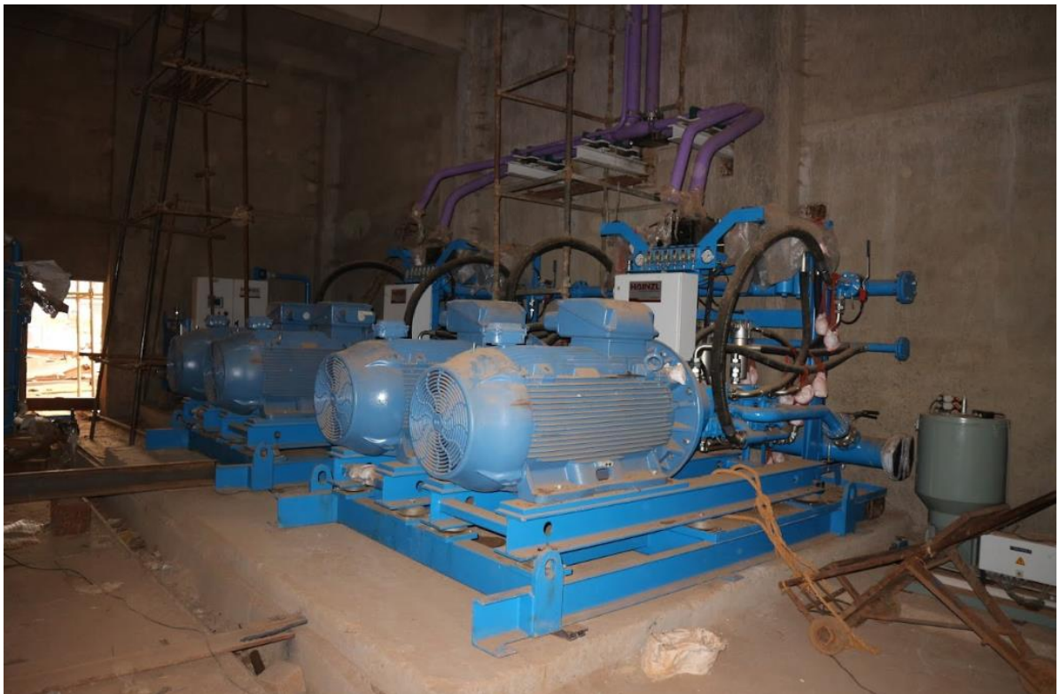
Hardline connected to be connected to the Hainzl HPU
