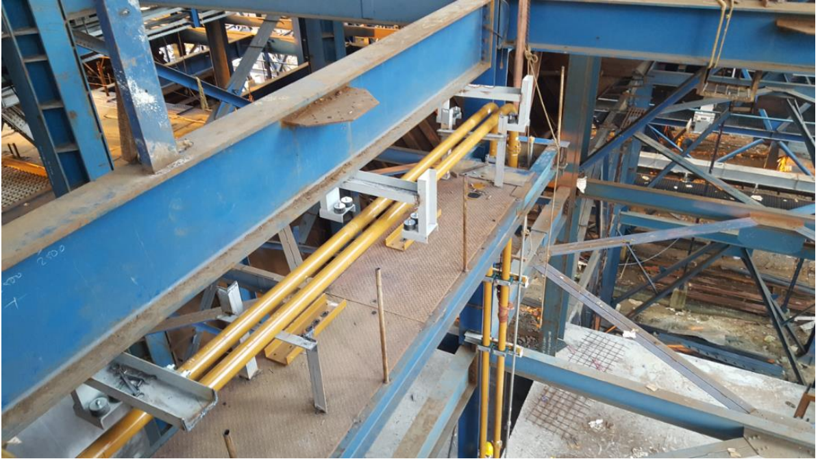
Hardline view above Pump Room
