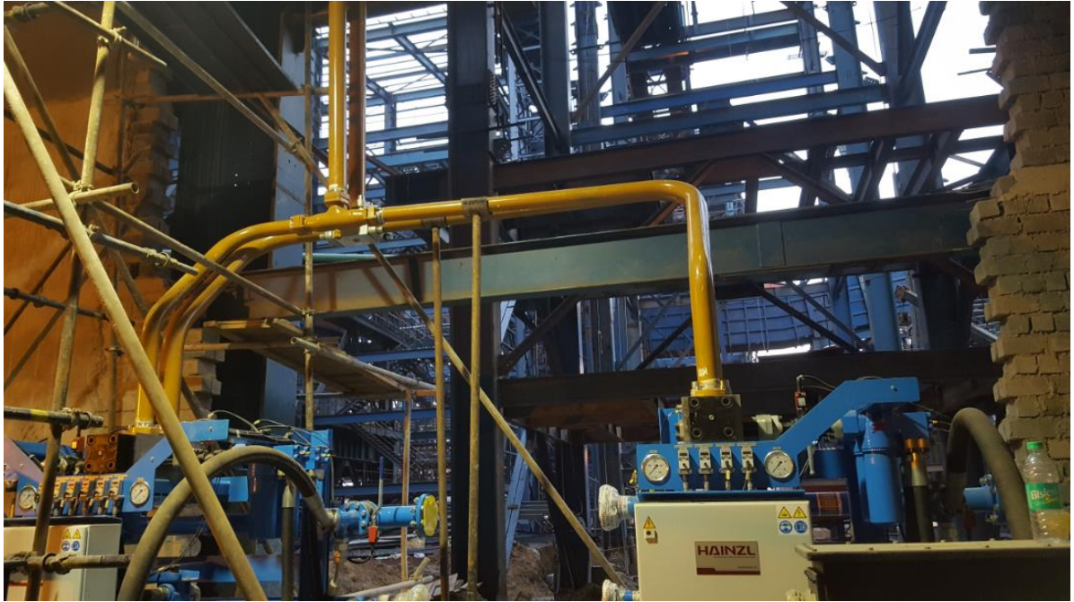
Hardlines mounted on the Hainzl HPU's.
