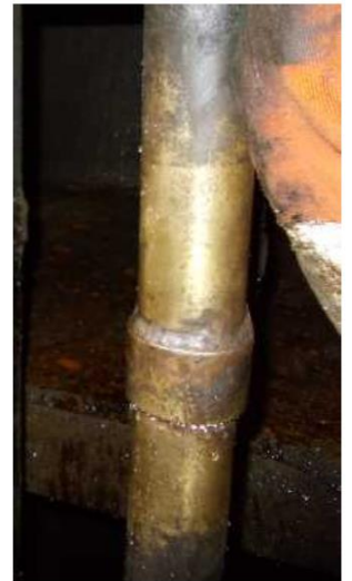
Tube and Leaking Fitting Exposed
