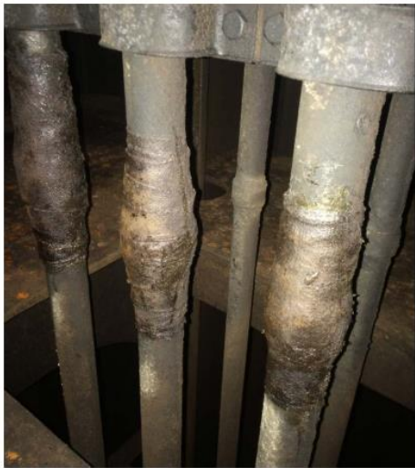
Leaking Joints before repair. They were wrapped with temporary repair band.
